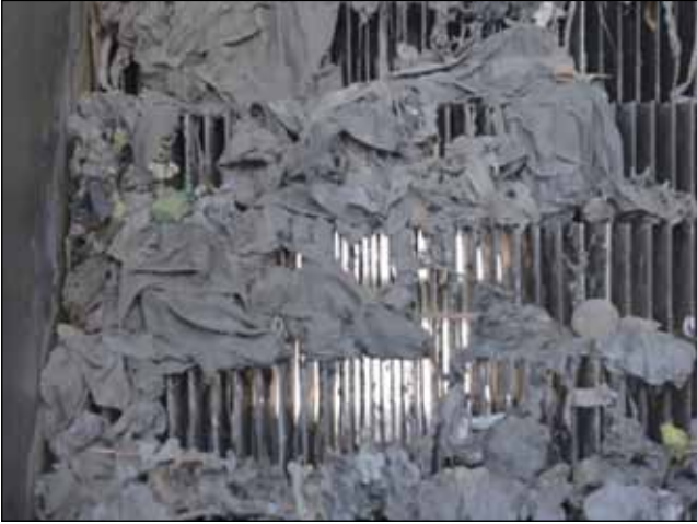
Wet wipes that end up in waste water treatment infrastructure can cause significant operational problems by clogging pumps and screens or blocking sewers
