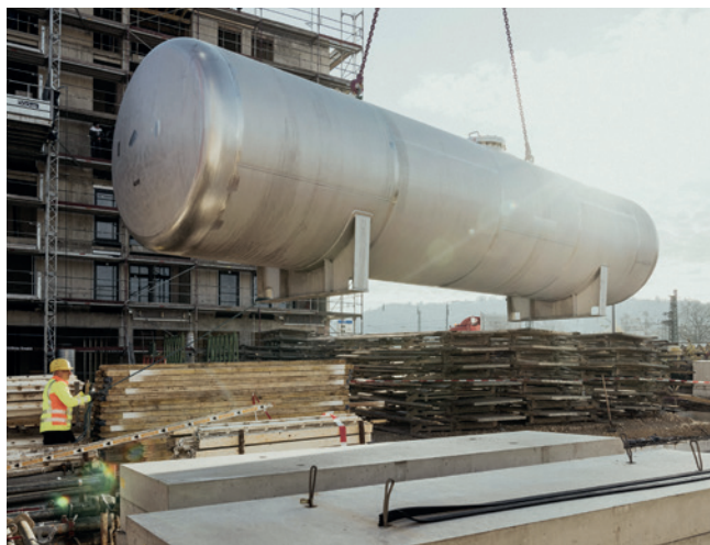
The H 2 storage reservoir is an essential component of the energy centre.
