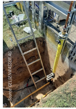
Connection of the H 2 injection plant to the existing gas grid
