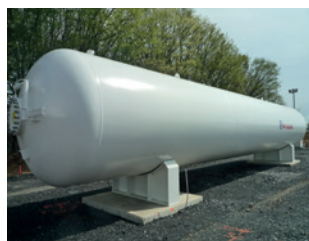
Hydrogen tank on the site in Holzwickede
