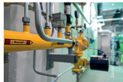
Through this pipeline, the green hydrogen enters the combustion chamber.
