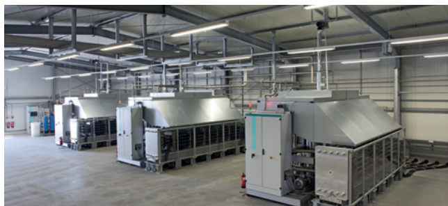
View into the electrolysis hall, where a total of three electrolyzers generate hydrogen.
